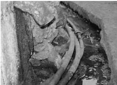
Plastic water pipes are laid along the drainage. They tend to crack and the water supplied is contaminated
